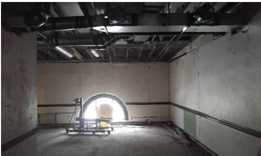
Central heat and cooling are being installed in The Cadet Lounge and other ROTC offices.
