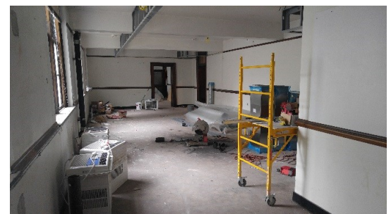
Old offices are becoming completely renovated to accommodate modern office standards while maintaining the historic look of the Armory.
