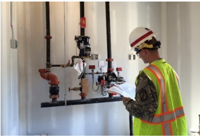
Cadet Corey Maisch inspects the fire suppression pump system at the Grundy National Bank site in Grundy, Virginia.
