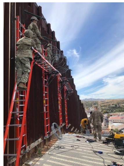
Engineer Soldiers place scaffolding on the US-Mexico border wall for later installation of concertina wire.
